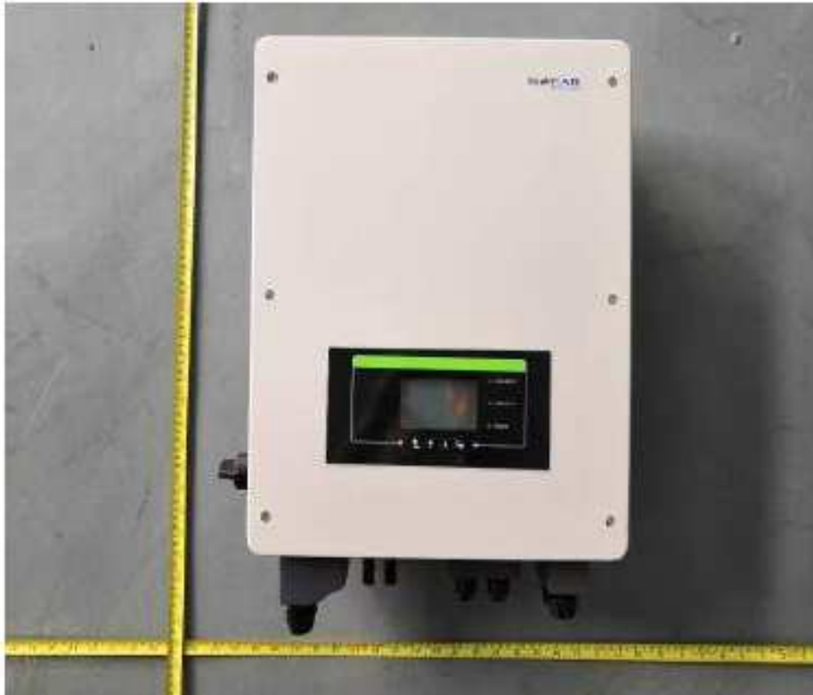
Front view of inverter
